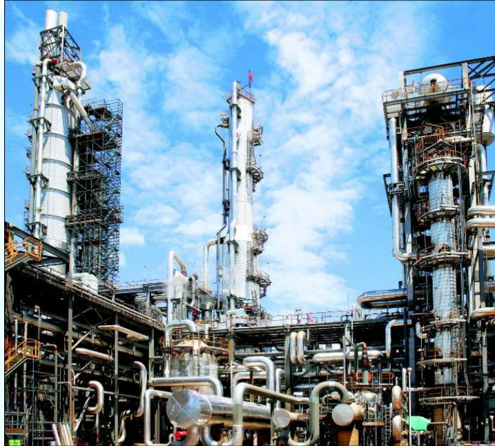
Feeding the demand: Gas diverted from Burrup Fertilisers plant helped generate power to meet the needs of Perth and Karratha
