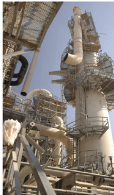
Construction work in progress on one of Qatargas 2's 7.8m t/y megatrains
