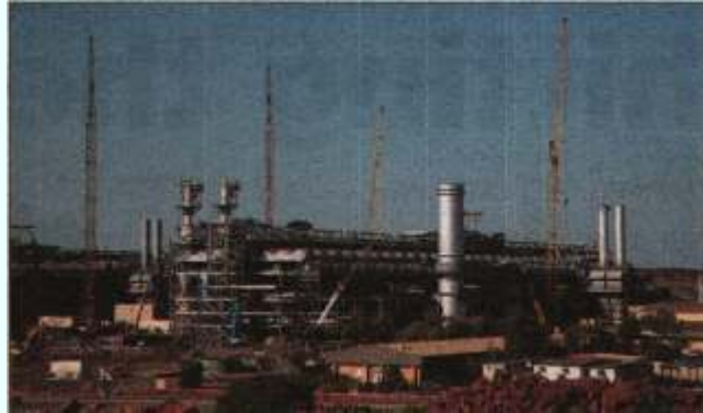
Woodside's new 'Train 5' installation is now operational at its Karratha Gas Plant on the Burrup Peninsula.
